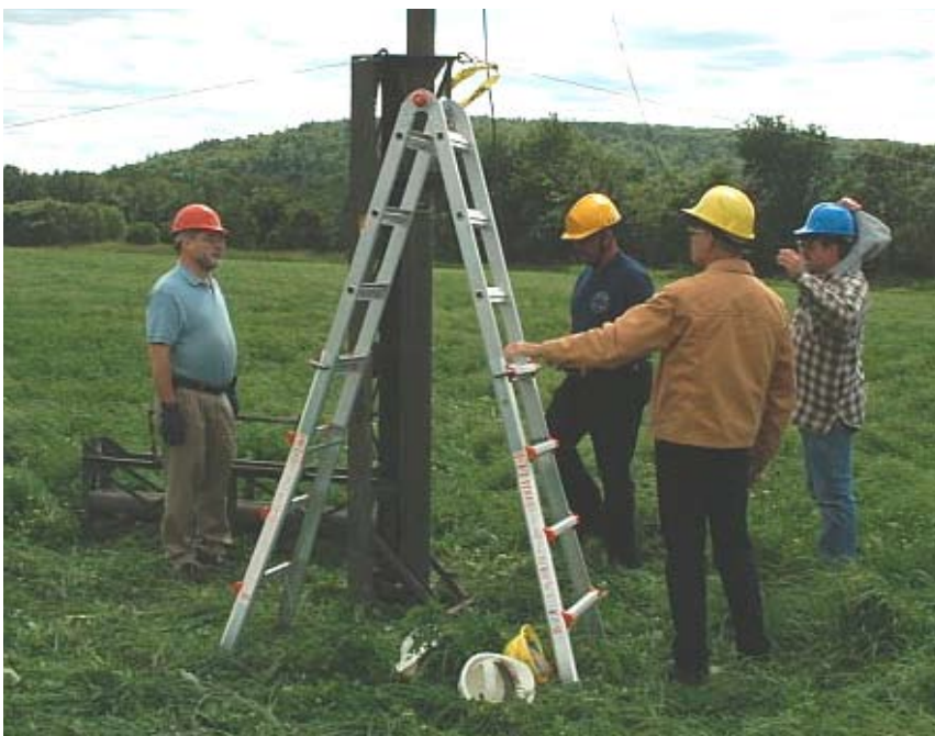
N1YMQ, K1DAN, KB1ELY and WB9MHI make short work of the last tower at Field Day
